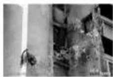
Damage to residential buildings in Karlovac in May 1991 during the Homeland War (photo: Zoran Mirković, source: ANKRA)
